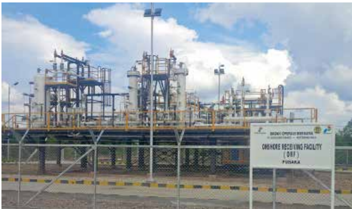
Onshore Receiving Facility (ORF), BOB PHE – BSP, Riau.
