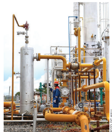
Gas Compressor Station, Bunyu Field, Kalimantan Utara.
