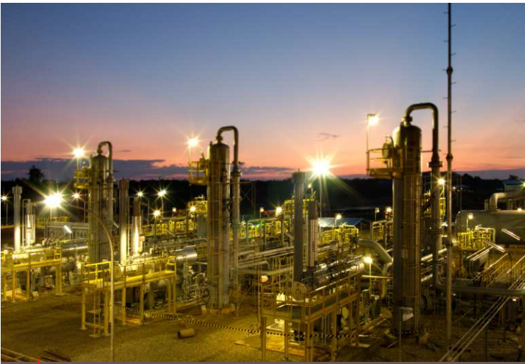
Kilang Geothermal Kamojang
